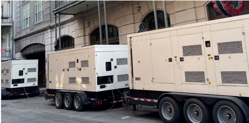
560kW Generator: Paralleling generators for load management expandability
